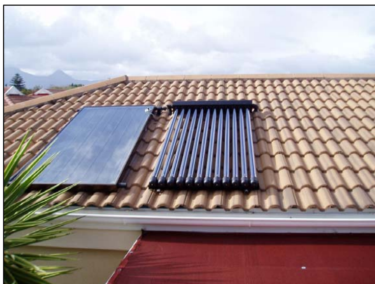
Figure 1: Solar collector placement.
